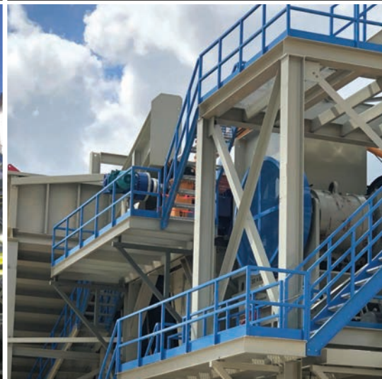
VULCAN WEATHERFORD Millsap, Texas 5062j primary station
