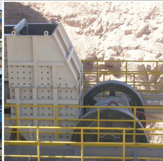
FRANKE COPPER MINE Antofagasta Chile Co 5062j
